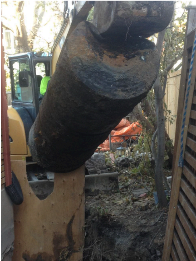
Environmental Professional Geoscientists conduct site assessments, manage removal of contamination source(s) (such as the leaking underground storage tank shown here) and manage soil and groundwater remediation to reduce hazard risks to the public. Photo courtesy of Hubley Geosciences Limited
